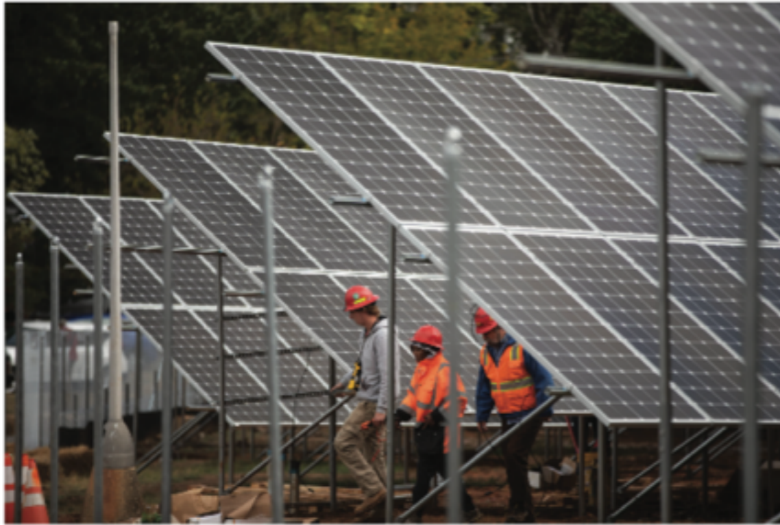
In 2019, workers installed more than 5,000 solar panels on Catholic Charities property in Northeast Washington, D.C. The solar array, the largest such project in the District of Columbia, was fully operational by the end of January 2020.
